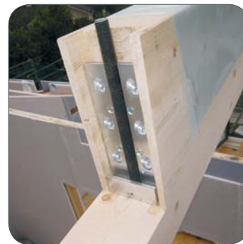
Concealed mounting on three sides by milling the secondary beam and visible mounting on main beam.
