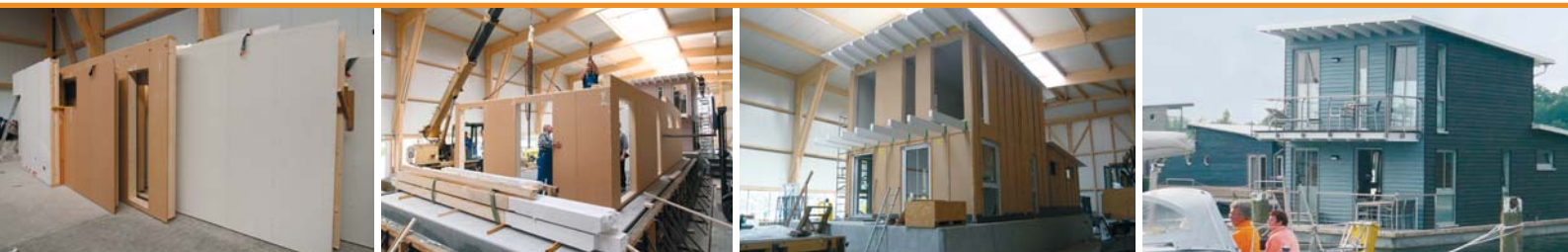
Construction of bathouses for the holiday water world „Im Jaich“ on the isle of Rügen (Germany)
